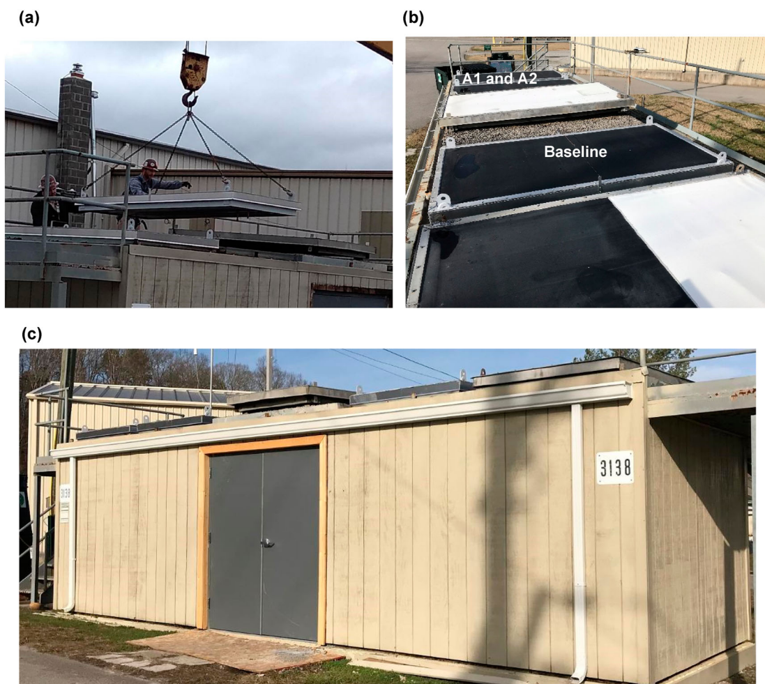
Figure 1. Field installation of TABE roof panels at the RTRA in Oak Ridge: (a) lifting panels into place and (b) after installation; and (c) exterior of the RTRA test facility.
