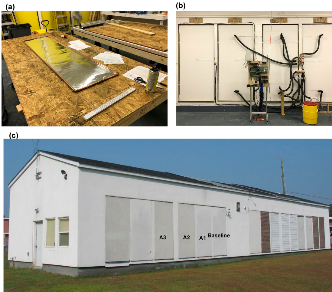
Figure 2. Field installation of TABE wall panels at the Charleston NET facility: (a) panel preparation and (b) panel installation; and (c) exterior of the NET facility.
